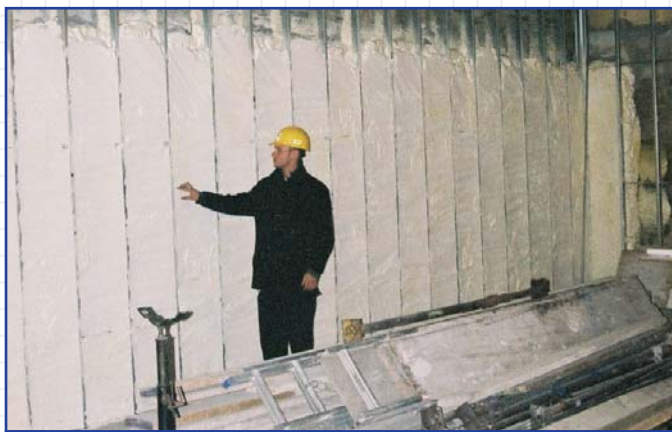
Penta Protective Coatings, Icynene Licensed Dealer in West St. Paul, Manitoba, sprayed Icynene® into the exterior walls of the building to protect the shell from a major source of energy loss – air leakage.
